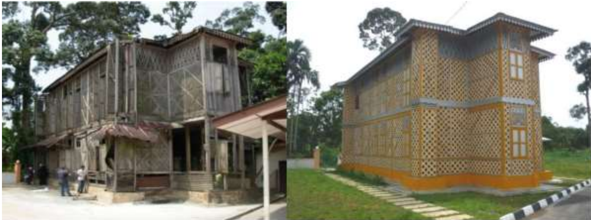
Figure 2.1. Kampung Kuala Dal Old Mosque, Kuala Kangsar before and after conservation in 2009. (Harun, 2011)
